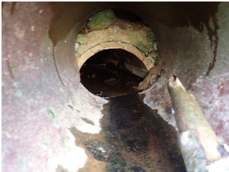
5. Interior view of the pipe opening in the right sidewall. Note the open joint and pipe displacement.
