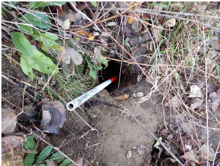
11. Several deep rodent burrows were noted in the canal slope.
