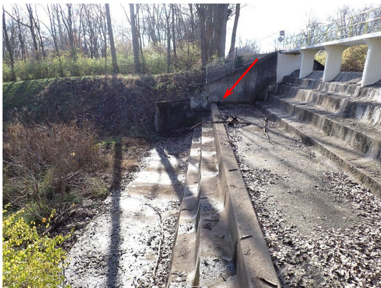
3. Principal spillway #1 outlet. Note the pipe opening (of unknown purpose) in the right sidewall.
