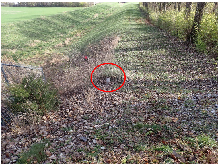
6. There is a standpipe of unknown purpose adjacent to the unknown piping through the sidewall.
