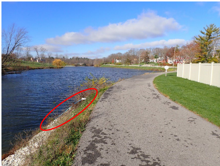
14. View of the dam crest. Note the hoses into a PVC pipe through the upstream slope.
