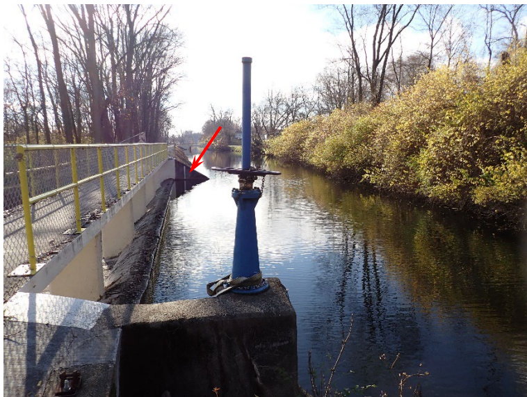
2. Principal spillway #1 inlet. Note the lake drain valve at the left end and the staff gauge at the right end.
